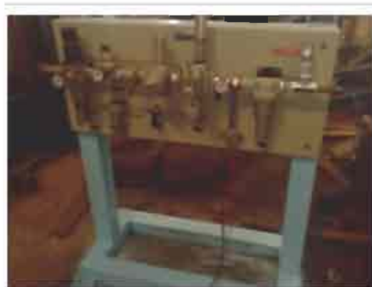
LPDC PNEUMATIC PANEL
