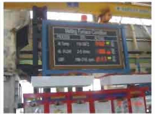
MELTING FURNACE CONDITION
