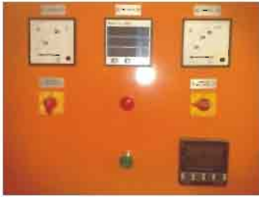
LPDC HEATER PANEL
