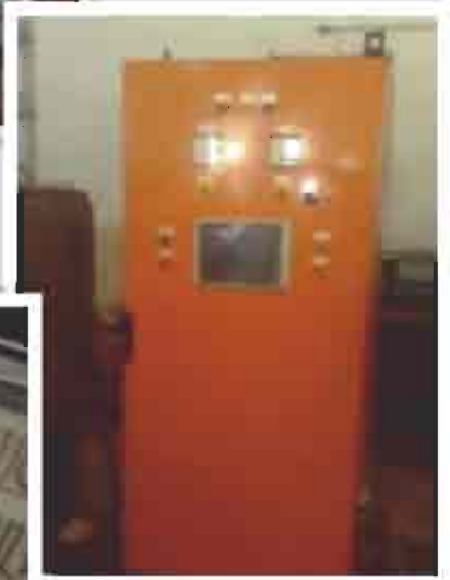
CONTROL PANEL OF LPDC
