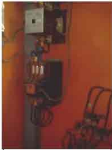
LPDC HEATER PANEL
